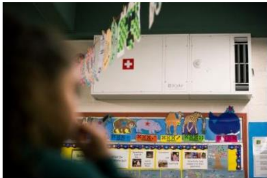
Air filtration system installed in an elementary school
