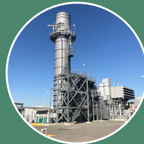
Rules Requiring Best Available Retrofit Control Technology (BARCT)
