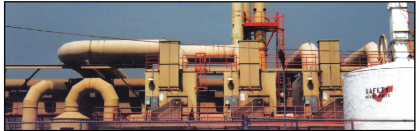
Collection of secondary lead oxide emissions using four FEF SERIES units.
