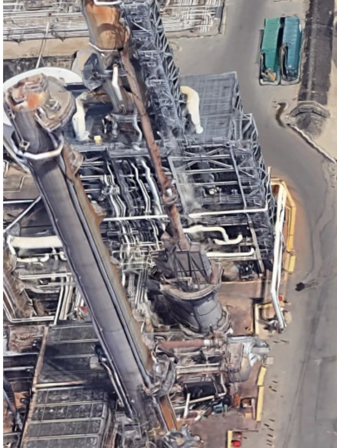
Figure 2-6. Relatively Open Access: Refinery Heater
