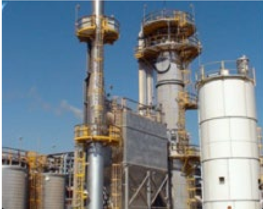
Figure 2-3. Sulfur Recovery Unit/Tail Gas Oxidizer
