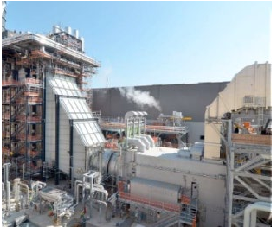
Figure 2-4. Gas Turbine with Heat Recovery Steam Generator
