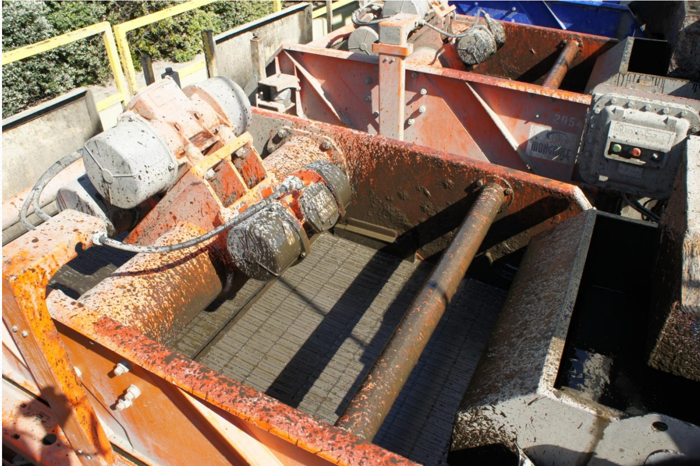
Drilling mud system
